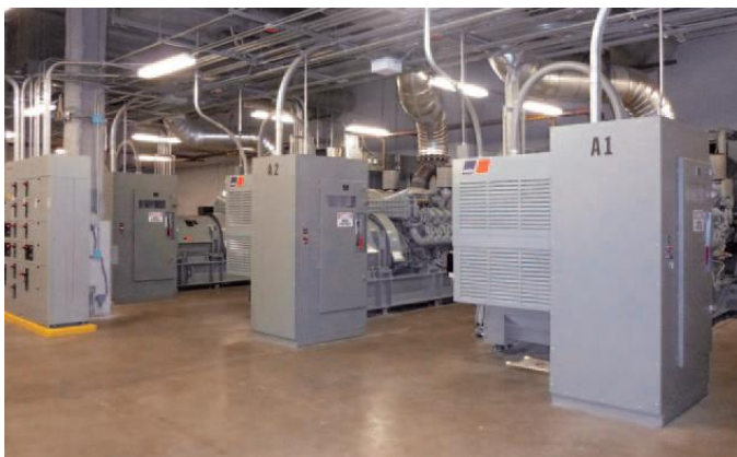
The medical center's emergency power system includes six 2,000 kW generator sets from MTU Onsite Energy.
