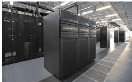
The COPT DC-6 data center uses a two-story design with the raised floor on the second story and the mechanical and air-handling equipment on the ground floor to maximize server rack space and improve cooling efficiency.
