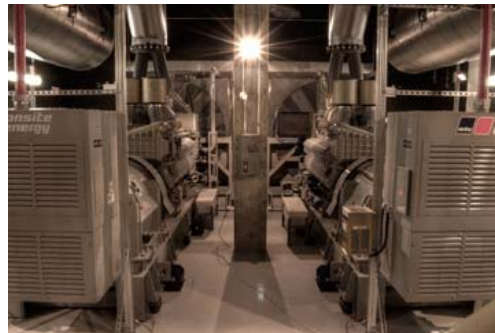
Two MTU Onsite Energy 3,000 kW generator sets inside Royal Jubilee's new energy center provide emergency standby power.
