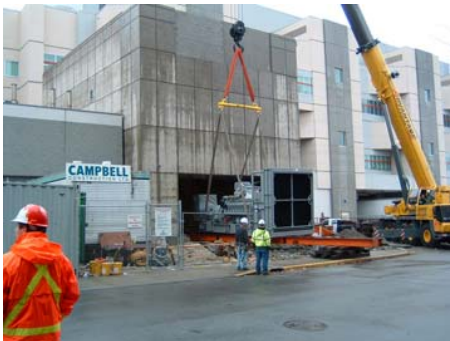
One of two MTU Onsite Energy generator sets powered by MTU 20V4000 engines is positioned into place at Victoria's Royal Jubilee Patient Care Center.
