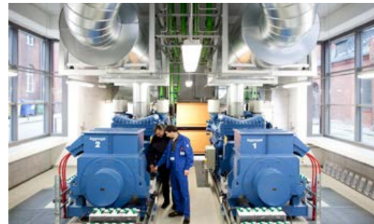
The two generator units are based on MTU type 12V 4000 G23 diesel engines with a combined electrical output of roughly 1,700 kVA and can be up and running inside ten seconds. (Picture: Rolls-Royce)
