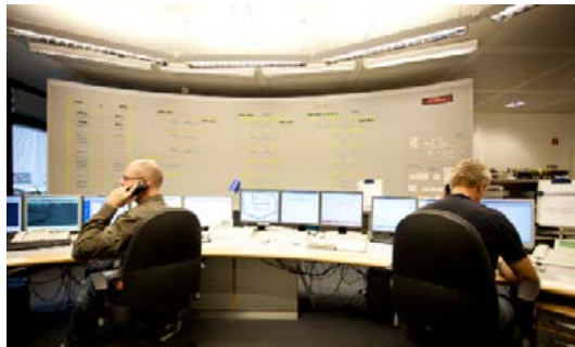
A look inside the technical control room of the Charité at the Campus Charité Mitte site, in the background the overview switch panel for the electrical supply of the Campus: From there the staff has everything in view. (Picture: Rolls-Royce)
