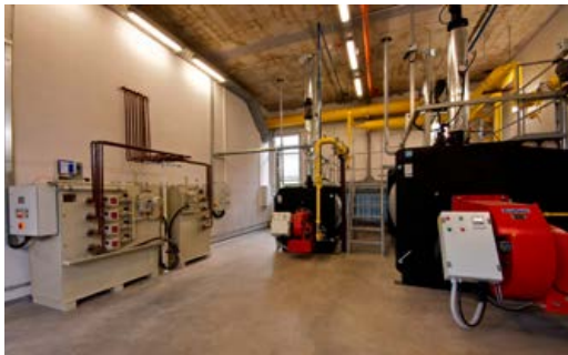
Daugavpils Siltums uses the exhaust heat from the generator sets to heat two additional water boilers. Holding 1,500 and 4,900 liters respectively, they are only operational in winter to handle unexpected peak loads. (Image: Baltic Marine Group)
