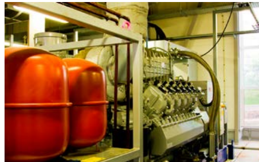
The compact heat modules. At the first Daugavpils Siltums site, each of the four generator sets of MTU Type GR 999 N5 produces 1 megawatt of heat and nearly 1 megawatt of electricity. (Image: Baltic Marine Group)
