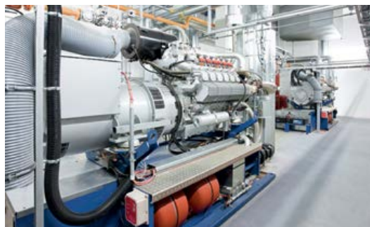
The two type GC 357 N5 CHP plants equipped with MTU Series 400 engines deliver around one megawatt of thermal and approx 700 kilowatts of electrical energy. (Picture: Marcel Mayer)
