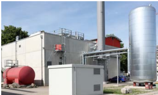
In order to handle the cogeneration module's higher electrical power, a 0.4/20kV transformer (seen in front) was set up in the combined heat and power station. (Picture: MTU/Ralf Dunker)
