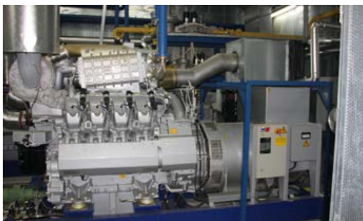
At the heart of the CHP plants in Belek are MTU Series 4000 gas engines with 8, 12 and 20 cylinders. (Picture: Rolls-Royce).
