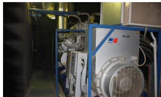
The CHP plant in the Kaya Palazzo Belek Hotel delivers 1,286 kWe/h of electrical and 1,124,240 kcal/h of total thermal power. It also delivers 1,094,000 kcal/h of total cooling energy. (Picture: Rolls-Royce)
