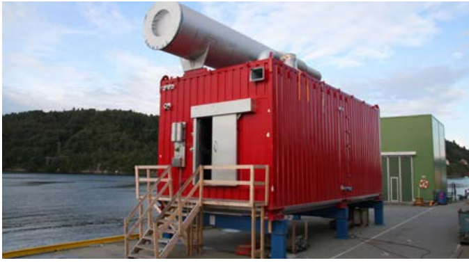
The MTU engines were installed in the fireproof containers for the fire extinguishing system at Frank Mohn and subsequently delivered to Statoil Hydro for installation on the Gjøa offshore platform. (Picture: Frank Mohn)
