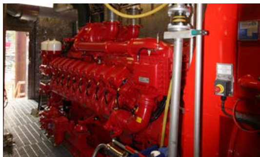
The pumps are driven by four MTU Series 4000 20-cylinder engines capable of 2,800 kilowatts each. (Picture: Rolls-Royce)
