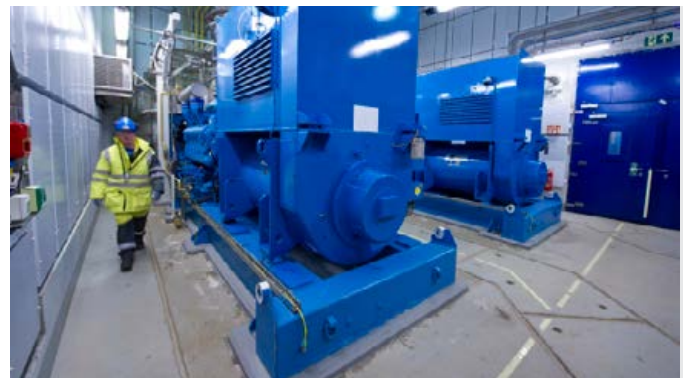
Interior view of the generator building with MTU gensets Type 16V 4000 G63. (Photos: Øyvind Hagen/Statoil)
