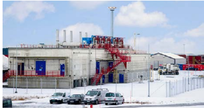
All MTU emergency gensets are housed in their own generator building on the Kårstø site. Rolls-Royce also supplied five horizontal core radiators with extremely low noise levels which were installed on the roof of the generator building. (Photo: Øyvind Hagen/Statoil)
