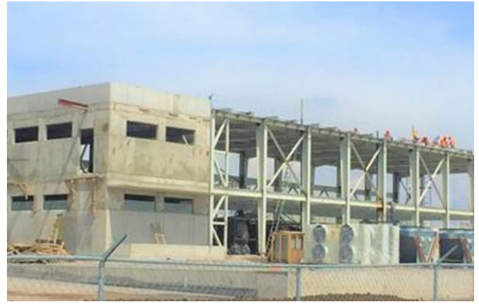
Example #3: Greenfield Food Industry Plant - Mexico
